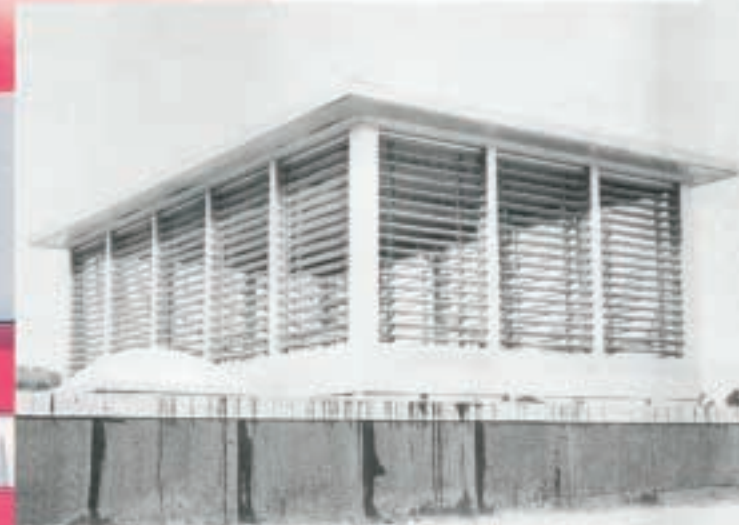
AIR INTAKE —The louvered penthouse located above the blower has motor operated adjustable blades controlled from the main instrument panel in the test chamber.
